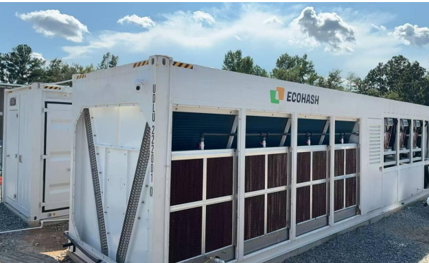
Evaporative Cooling Section
